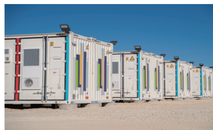
Texas, USA 226MWh Frequency Regulation
