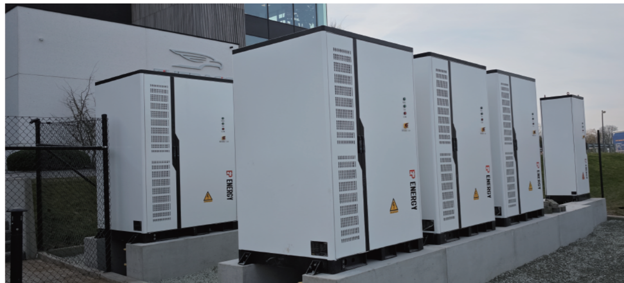
Willebroek, Belgium C&I BESS
